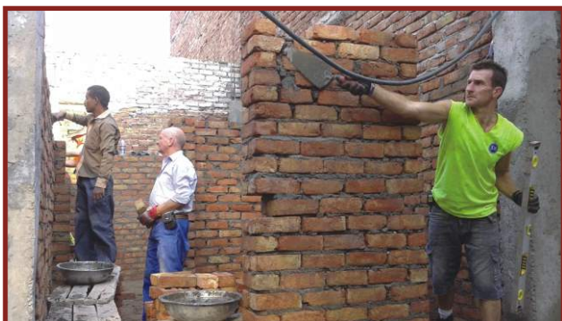
The Ballymena builders constructing the house of Rajendra Yadav in Saavda slum colony
